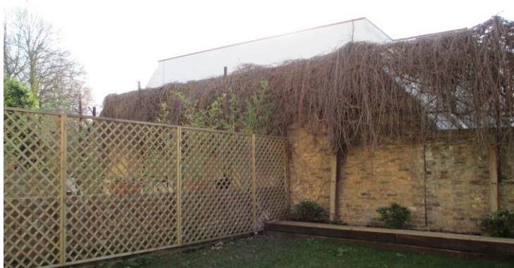
Photograph 6: The eastern flank wall of the school from a Stonefield Street garden
